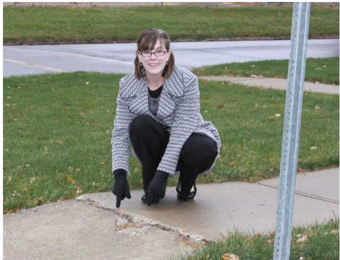
Sarah LaBrune-Jongeling, SIMPCO community development staff, inspects a cracked and bulging sidewalk.
